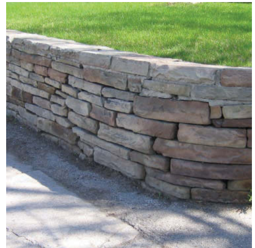
Figure 4.29 The existing stone wall on King Road in King City is a wonderful means of transitions heights. A more durable natural stone retaining wall product should be used to achieve the look and feel of the wall shown above.
