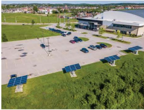
Solar panels at the Trisan Centre in Schomberg
