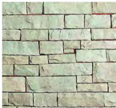
Figure 4.26 Stone is a recommended high quality construction material that is also recommended
